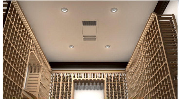
* Front grille and mounting bracket have been painted to match the ceiling
