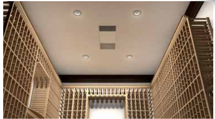
* Front grille and mounting bracket have been painted to match the ceiling
